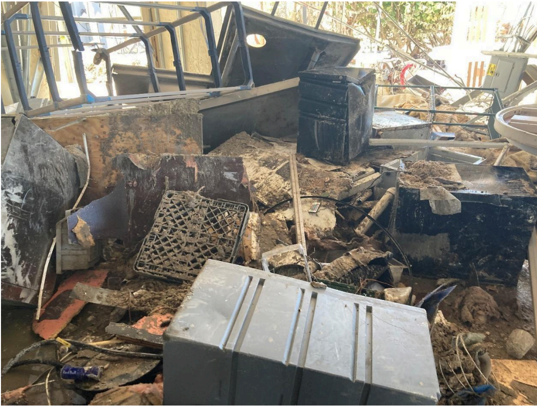
Damage to restaurant in Vanderbilt Beach caused by storm surge from Hurricane Ian (NWS Storm Survey picture)
